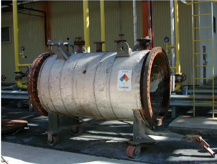
Figure 3. KD-502 polymer catch tank (actual vessel with one cover removed).
