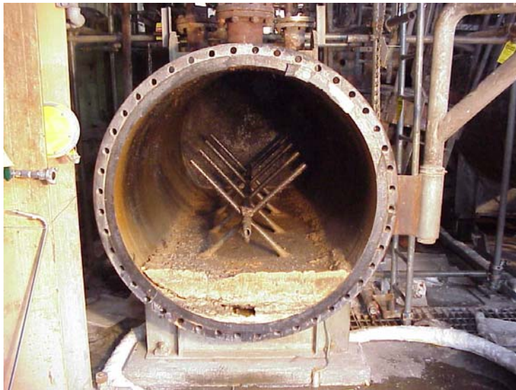
Figure A-3. Reactor knockout pot with internal frame visible.
