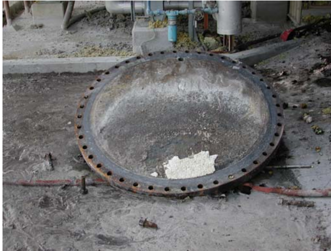
Figure 6. Polymer catch tank cover.
